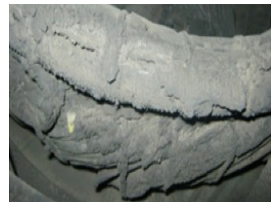
Typical deposits on an alternator used in a tropical industrial environment (palm oil refinery)
